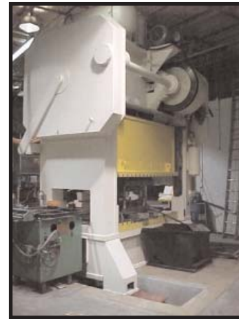
Press installation at Jade Corporation in Southampton, Pennsylvania
