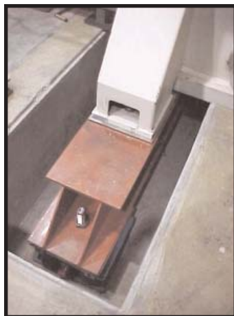
Close-up of the outrigger, press foot, and isolator
